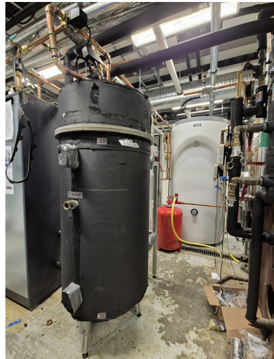
Figure 1: Thermal energy storage subsystem of the HESS (Stockholm, Sweden)
