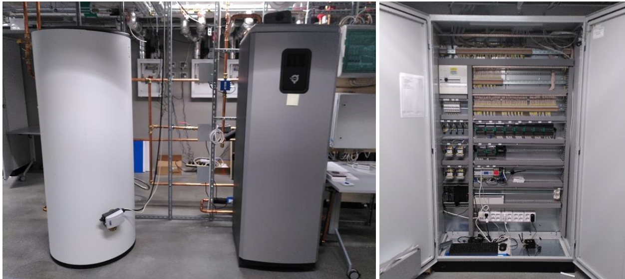
Figure 10: (From left to right): Water tank, heat pump, and BMS at the KTH Live-in Lab.
