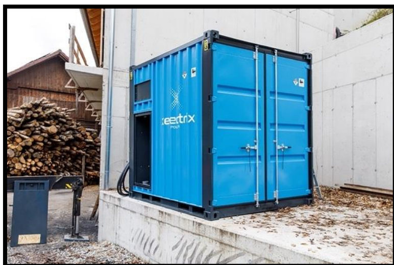
Figure 7: Xeectrix storage system (80 kW/140 kWh) in Gasen.
