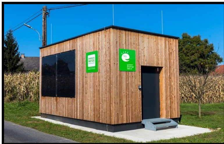
Figure 8: "Urban-box" with battery energy storage system (100 kW/100 kWh) in the municipality of Heimschuh.
